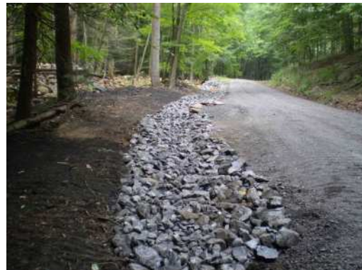
Limestone Lined Swale to treat runoff
