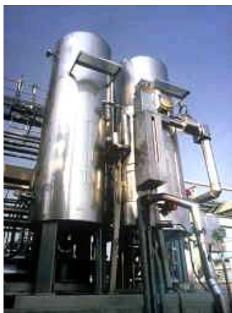
A typical Macro Porous Polymer Extraction System Installation.
