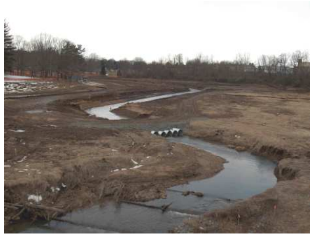
Angelica Park Stream Restoration Project, Reading, one of the tours from the Schuylkill Watershed Congress
